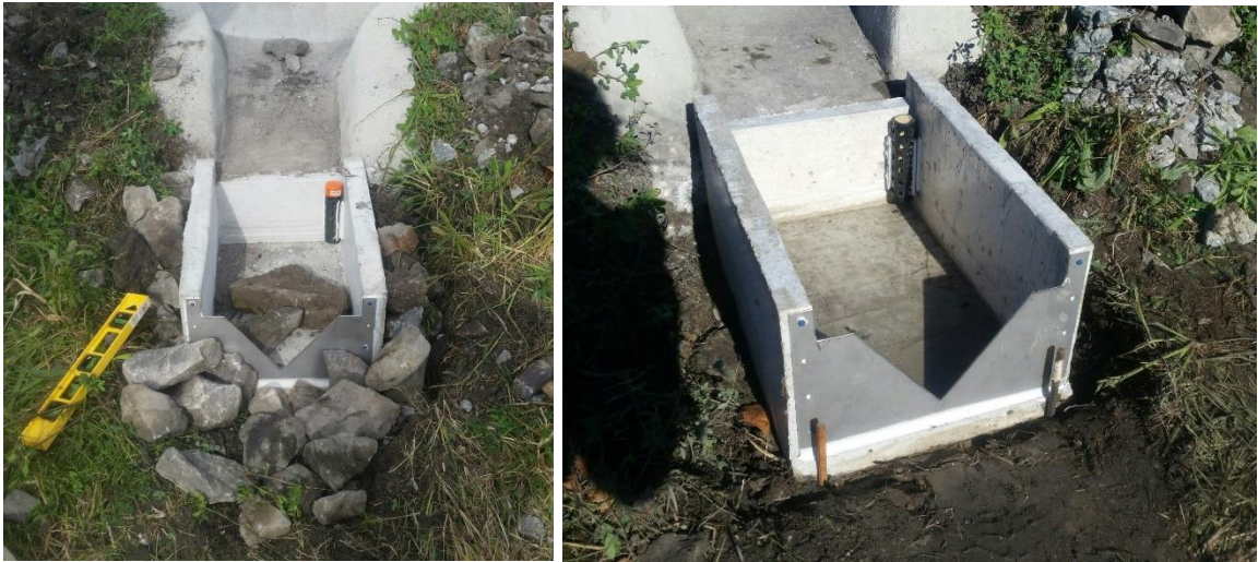
Figure A-2: Influent weir installed at curb inlet of the East bioretention system
