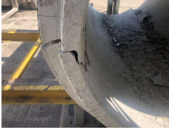
Figure 3.10-Flexural Cracking Causing Plastic Hinge in DC RCP.
