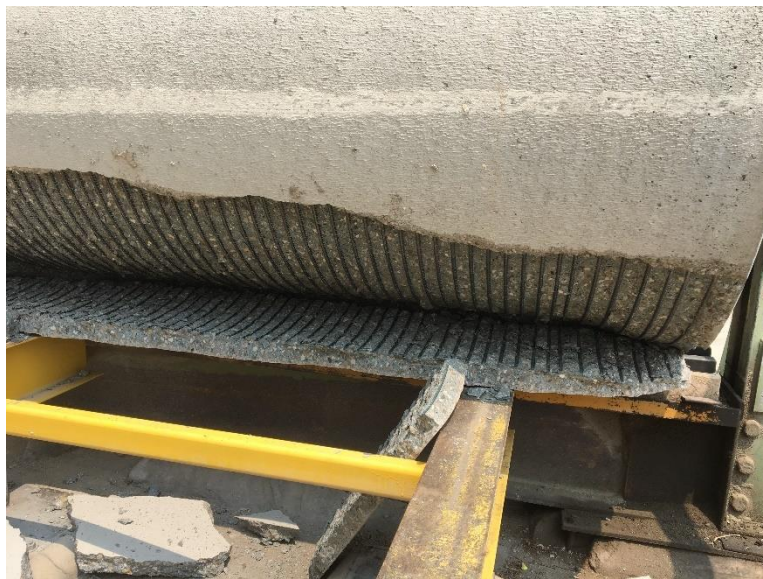
Figure 3.15-Major Concrete Slabbing in Sample E24.
