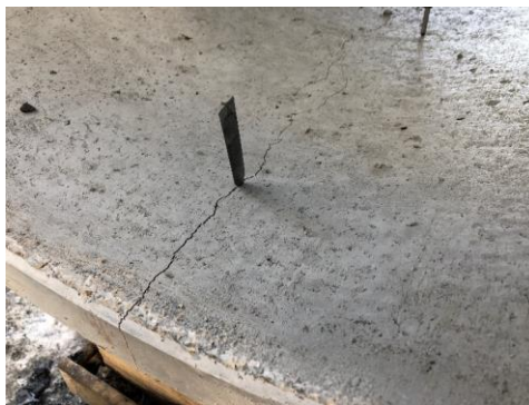
Figure 2.2-Leaf Gauge Measuring 0.3 mm Crack.
