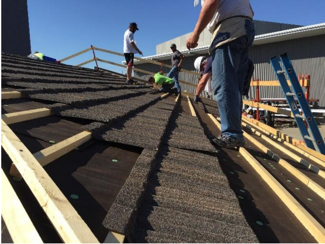
Figure 3.8: Photograph of the installation of the metal panels on the test building at IBHS.
