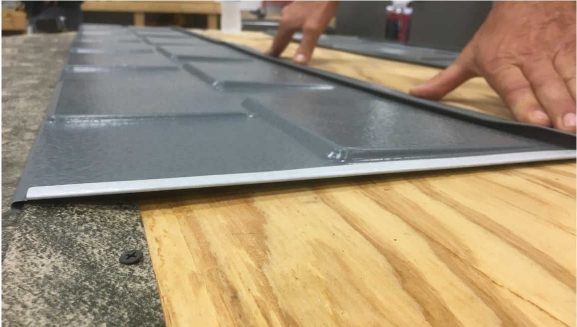
Figure 3.12: Photograph of metal shingles being installed on to a flat surface, demonstrating lap joint locations, and cavity details.
