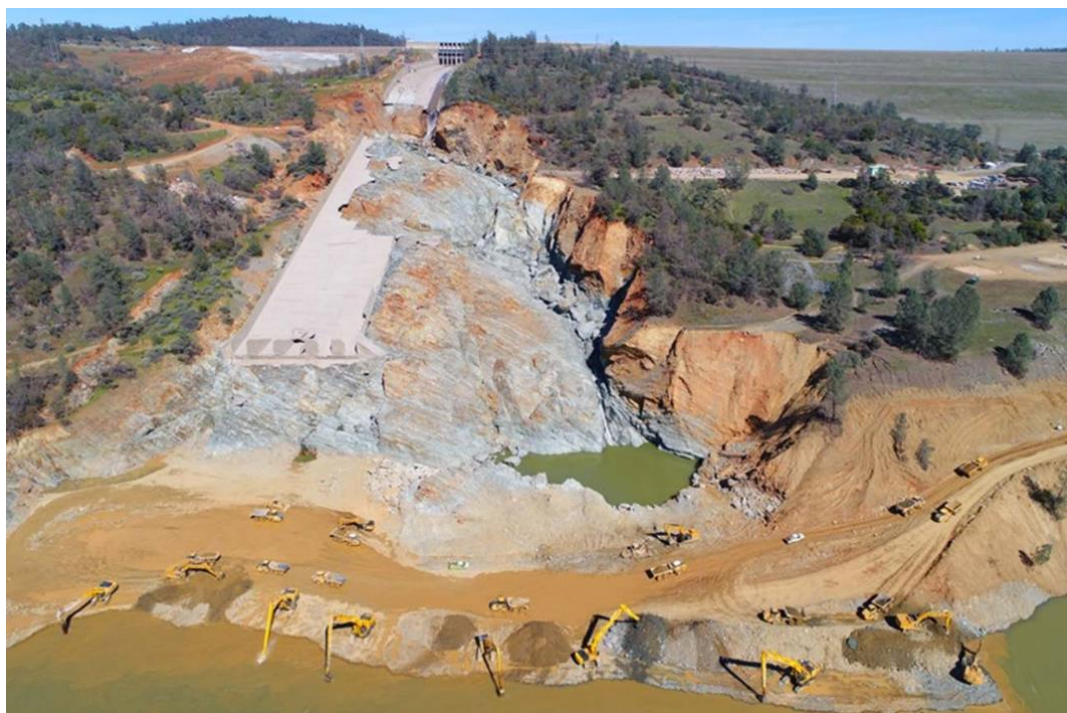
Figure 1-14: Oroville spillway chute after incident (France et al. 2018)
