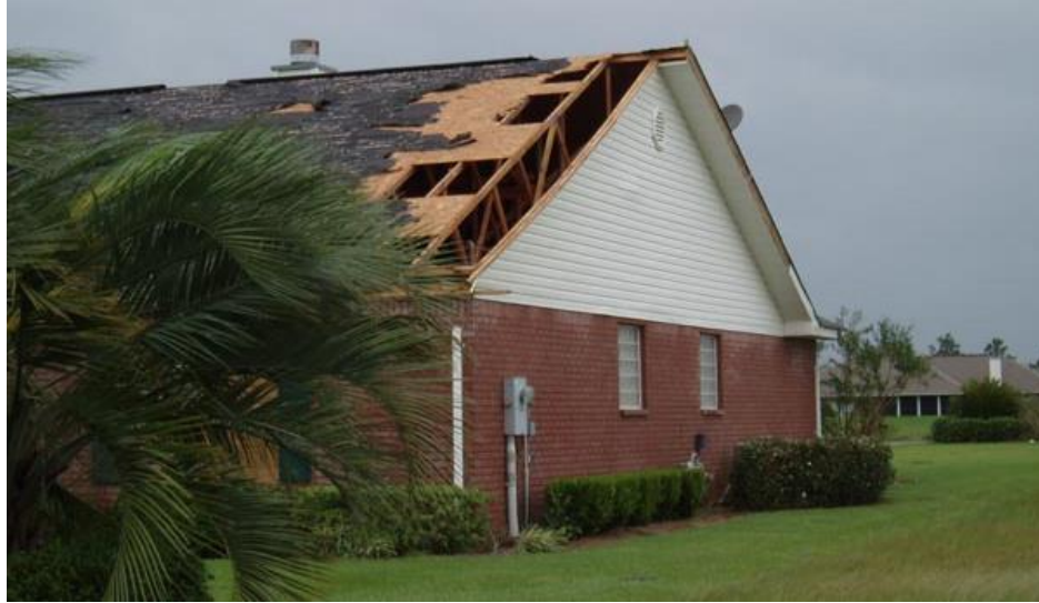
Figure 1.2: Failure of roof sheathing near the end gable truss.
