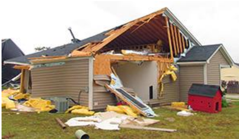
Figure 1.3: Failure of roof truss connections.
