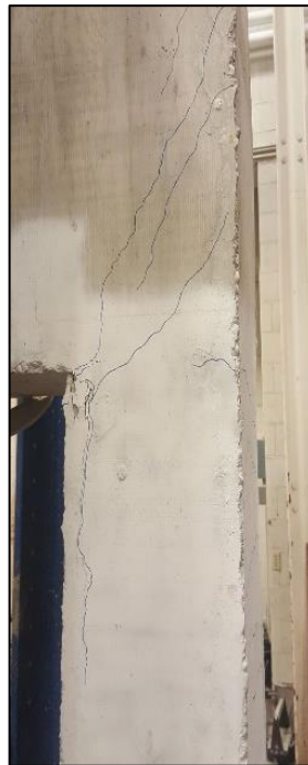
Figure 4.14: Typical Failure Mode of Column C1
