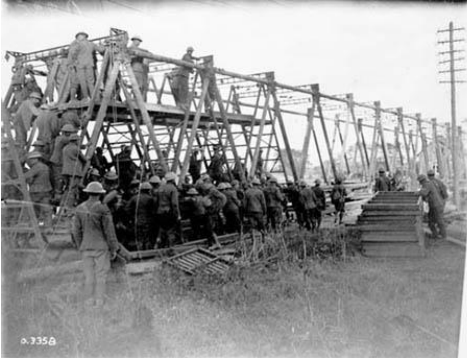
Figure 35 – Canadian Engineers Constructing a Bridge across Canal du Nord, during the Advance east of Arras, September, 1918 - LAC/PA-003456, taken from: http://www.veterans .gc.ca/eng/remembrance/history/first-world-war/last-hundred-days?filter=range&start=41
