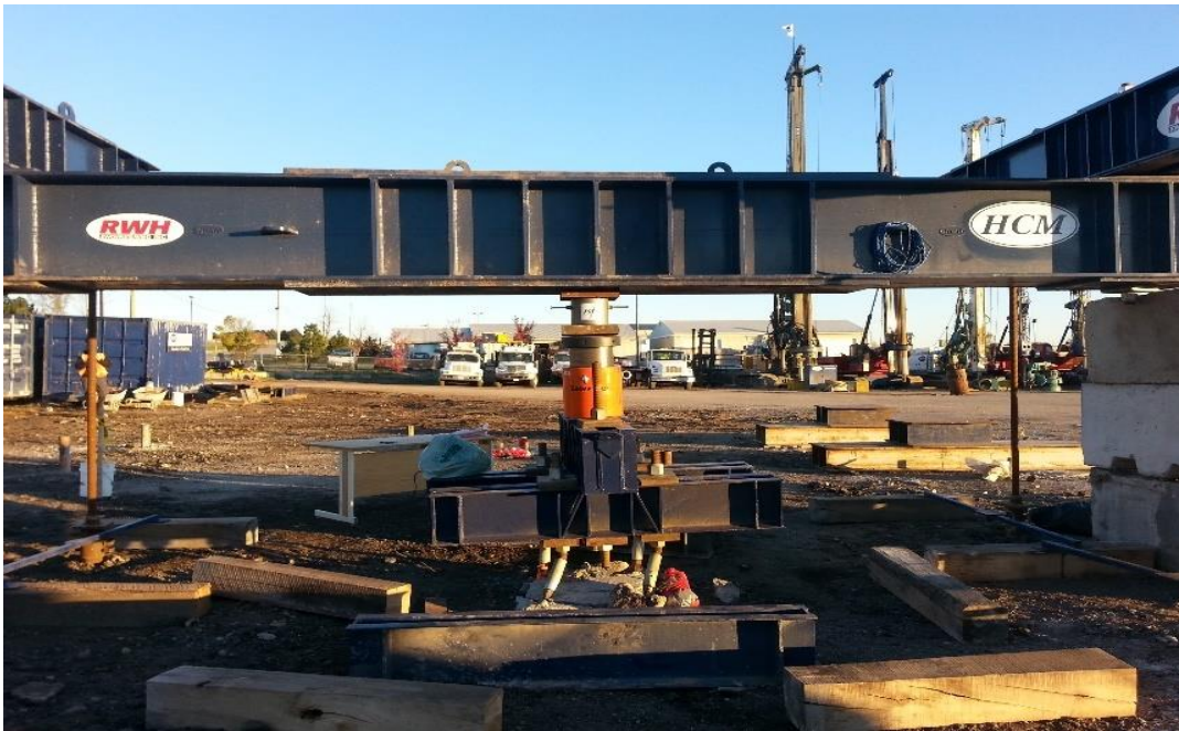
Figure 4-7 Structural failure of loading bar for MPG1
