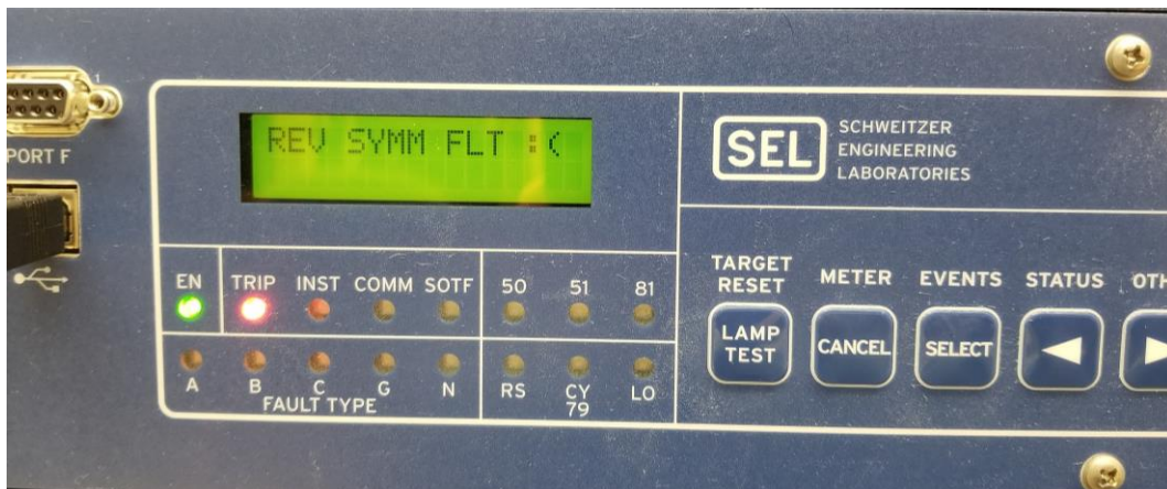
Figure 4.6 Front panel screen of SEL-351 detecting the reverse symmetrical fault.
