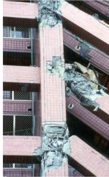
(b) Close up view of the failed BCJs
