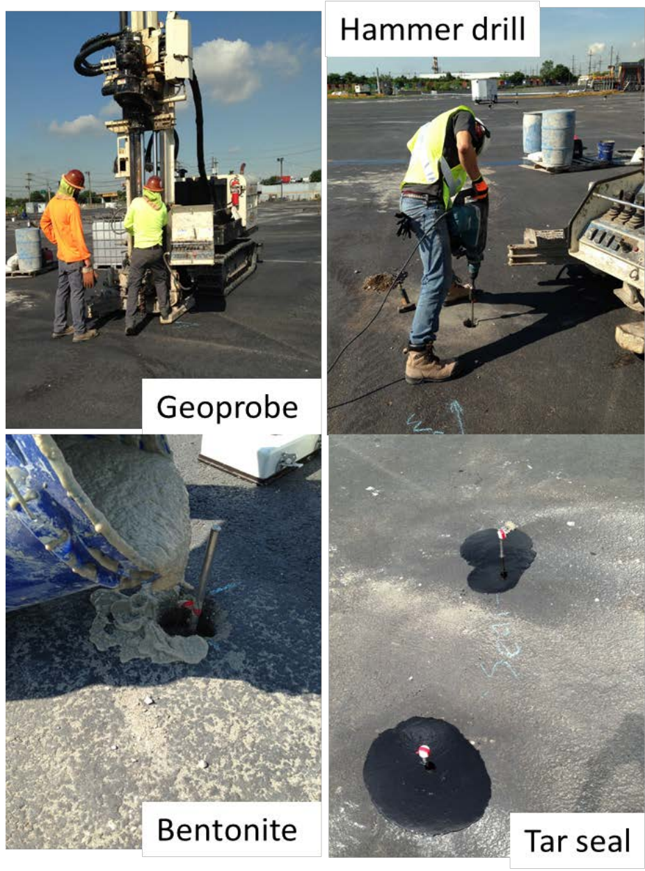
Figure B-2. Details on the installation of the ERT electrodes using geoprobe and hammer drill.
