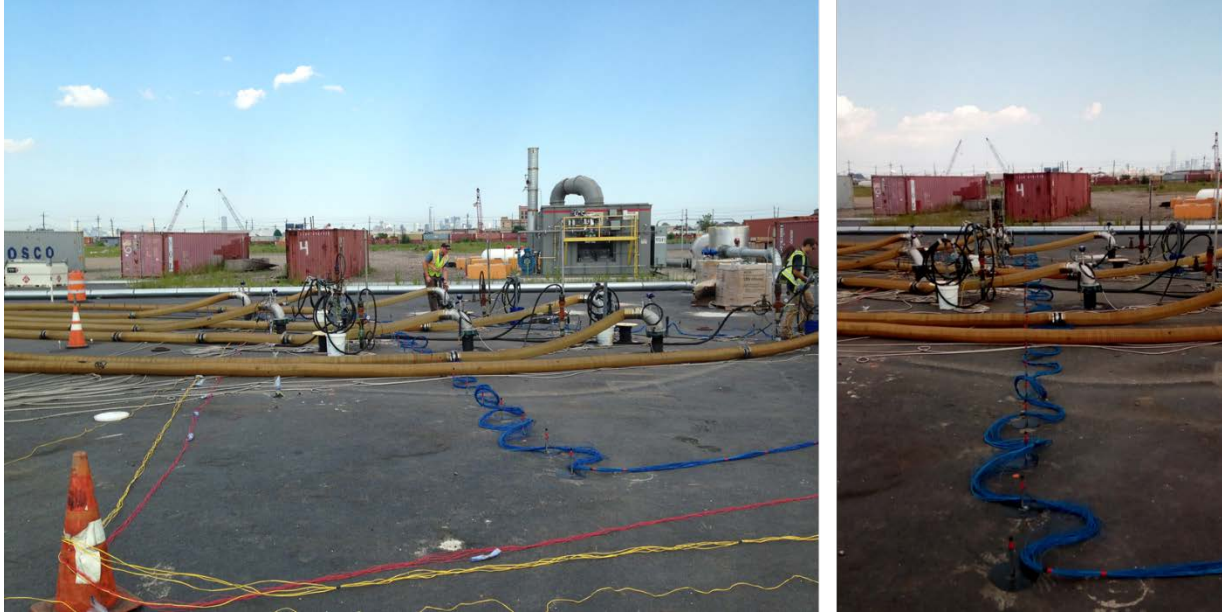
Figure B-3. Details on the installation of the ERT for the shallow cell.
