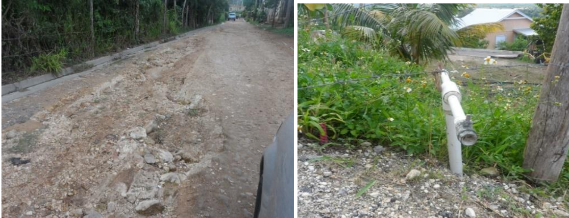
Figure 5.8: Infrastructure inequalities: Unpaved Roads and Lack of water pipes
