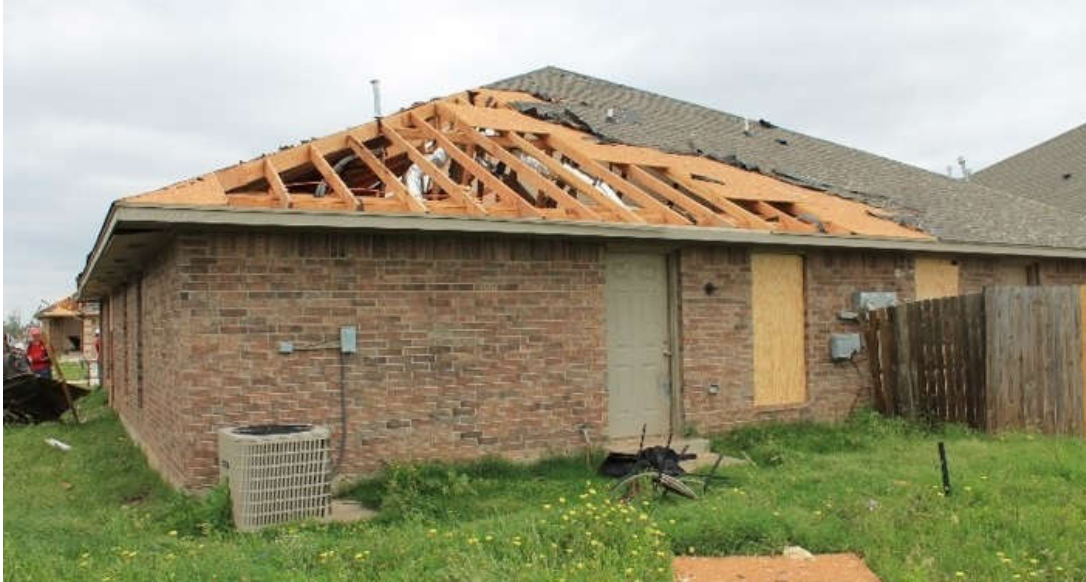
Figure 1-1: Example of roof sheathing failure, corresponding to DOD-4 (Image provided by Dr. David Prevatt of University of Florida)
