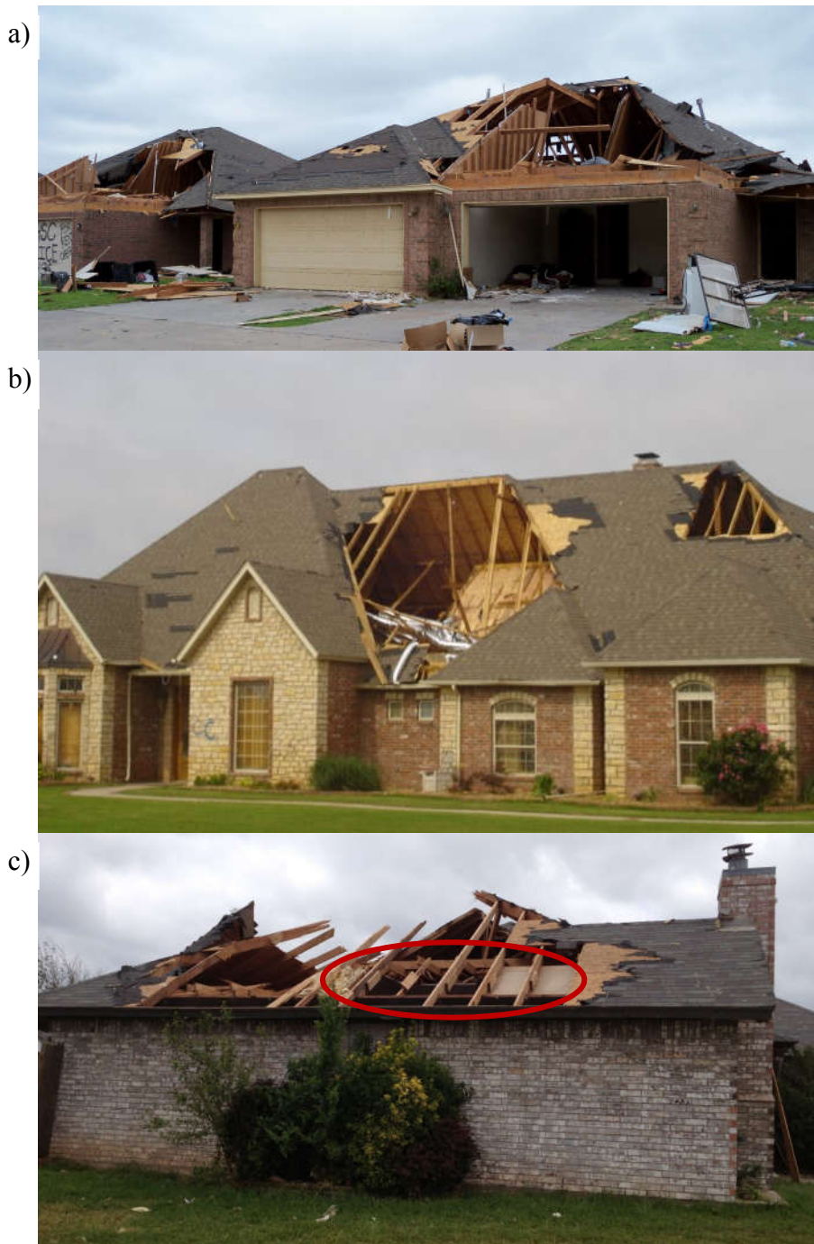
Figure 1-4: Hip roof failures in Moore, OK following the EF5 Tornado of May 21, 2013. a) Framing failure of similar, neighboring hip roofs b) Framing failure of steep, stick-frame hip roof c) Hip roof displaying material failure of the wood framing members (Images provided by Dr. David Prevatt)
