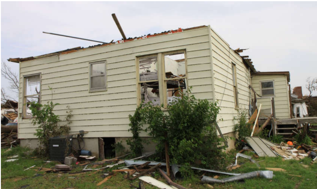
Figure 1-2: Example of roof-to-wall connection failure, corresponding to DOD-6 (Image provided by Dr. David Prevatt)
