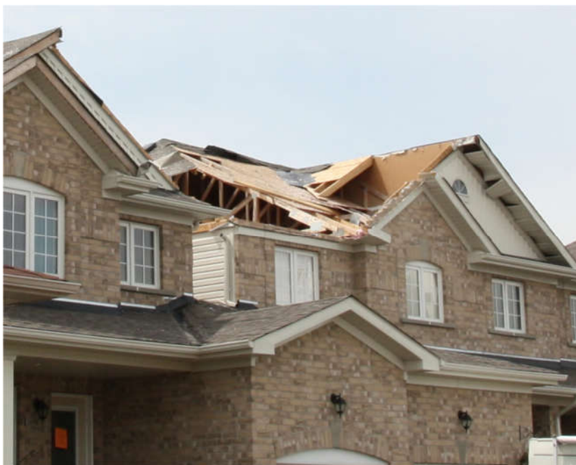
Figure 1-3: Partial hip roof failure observed following EF2 tornado in Angus, Ontario, June 2014. (Image provided by Dr. Greg Kopp)
