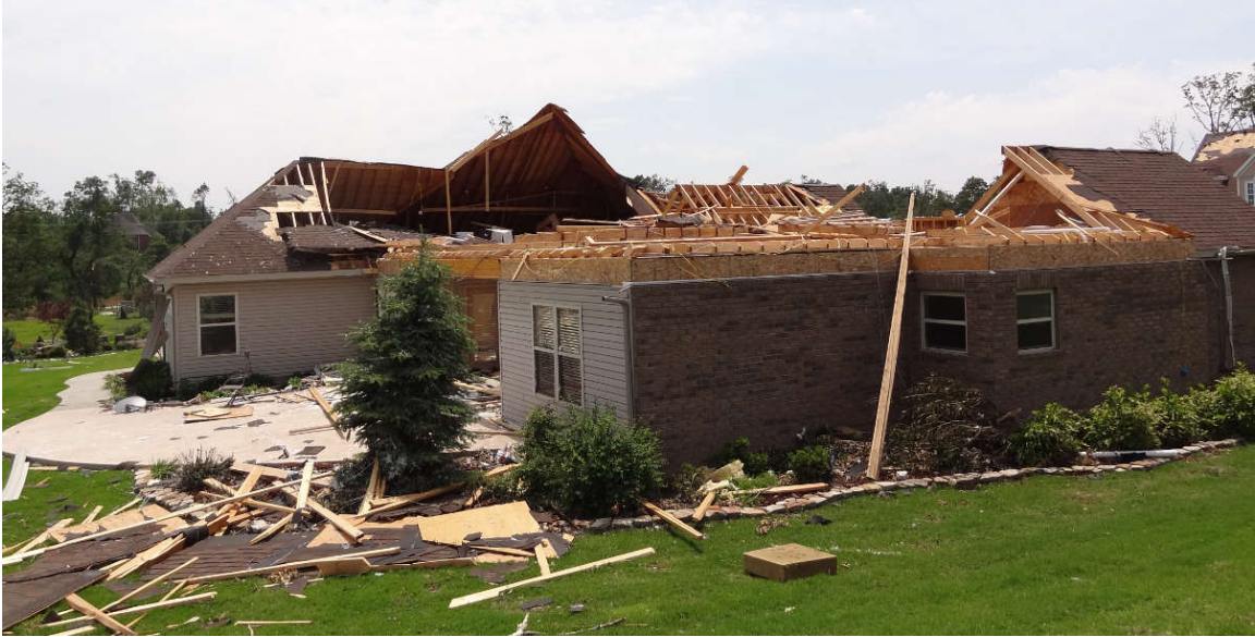
Figure 4-4: Partial stick-frame, hip roof failure with ceiling joists intact (Image provided by Dr. David Prevatt)
