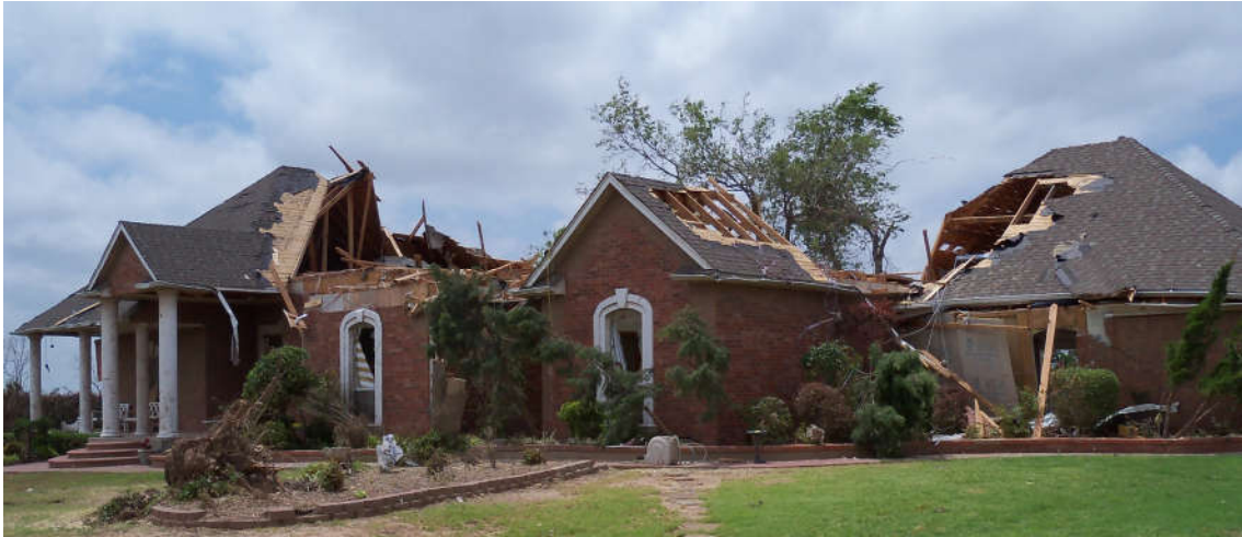
Figure 4-3: Failure of stick-frame roof with irregular roof shapes (Image provided by Dr. David Prevatt)
