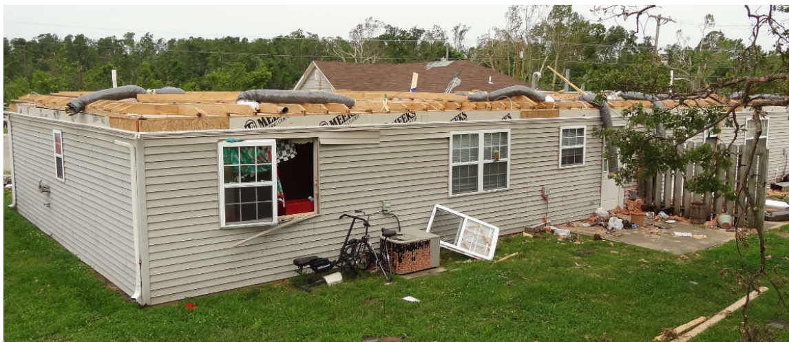
Figure 4-5: Loss of the entire surface of a stick-frame hip roof with intact ceiling joists (Image provided by Dr. David Prevatt)
