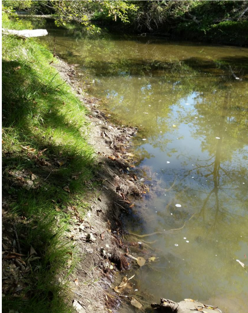
Figure 52: Spencer Creek Exposed Banks
