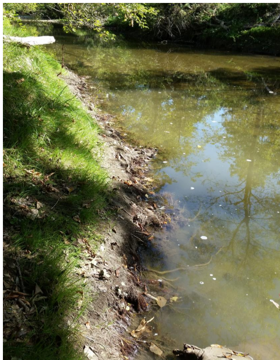
Figure 22: Spencer Creek Exposed Banks
