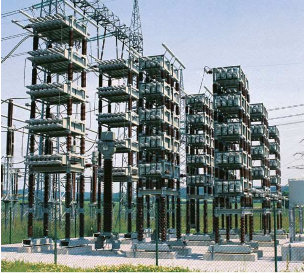
Figure 1.1: High Voltage Shunt Capacitor Banks (Scale Illustration).
