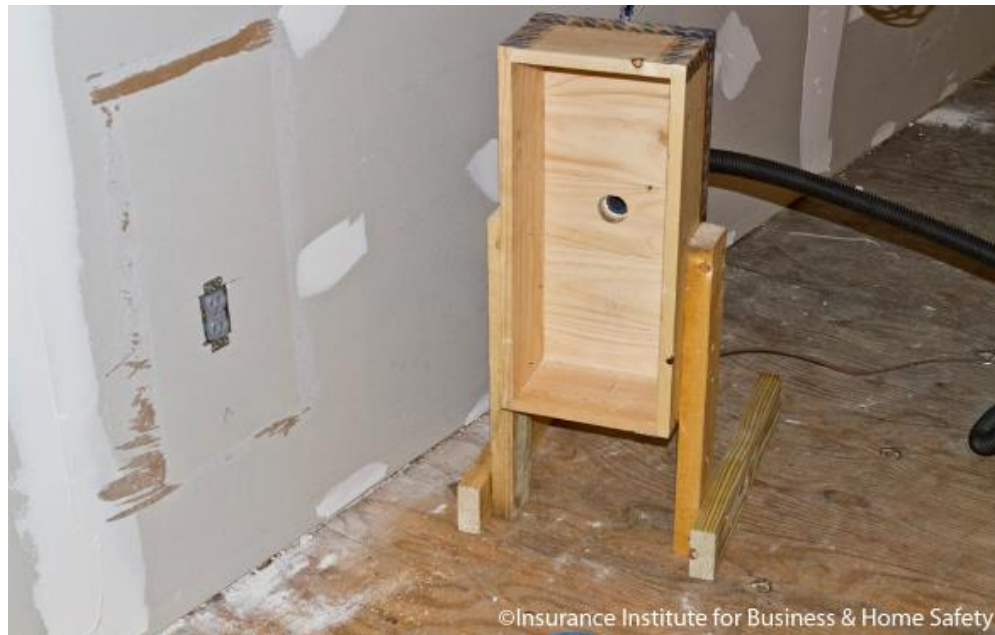
Figure 83: Typical electrical outlet with cover removed and ready for airbox mounting
