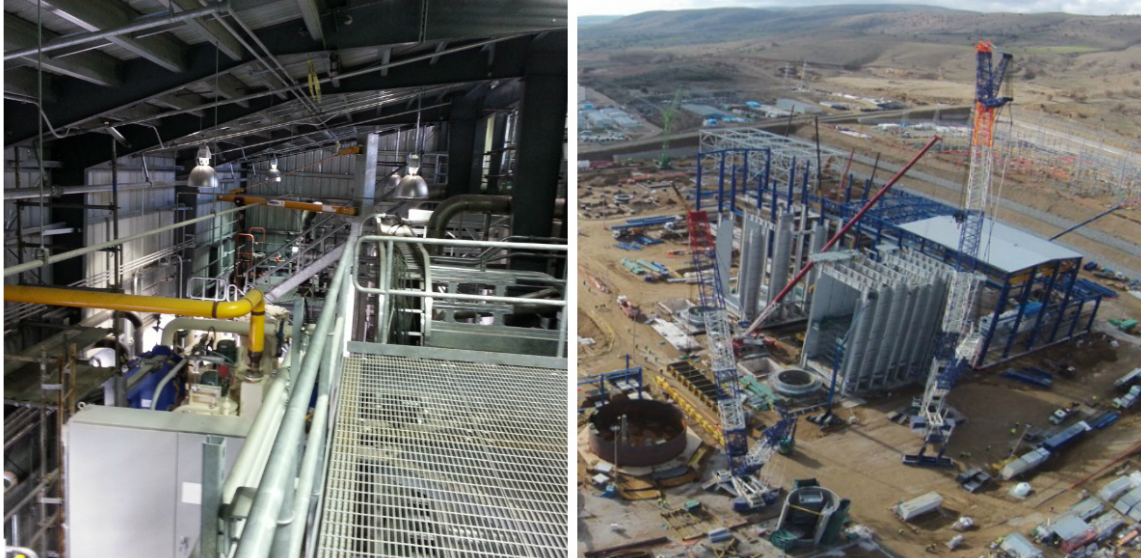
Fig. 2-4 Complex PEB Projects in energy generation industry (left inside a complex project, photo taken by author, right Outside a complex PEB project[39])
