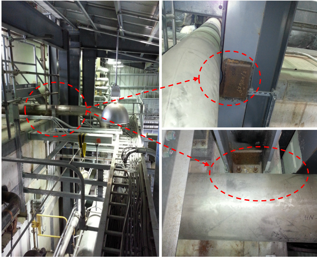
Fig. 2-5 Clashes detected at the construction phase of a PEB project in the absence of BIM implementation.
