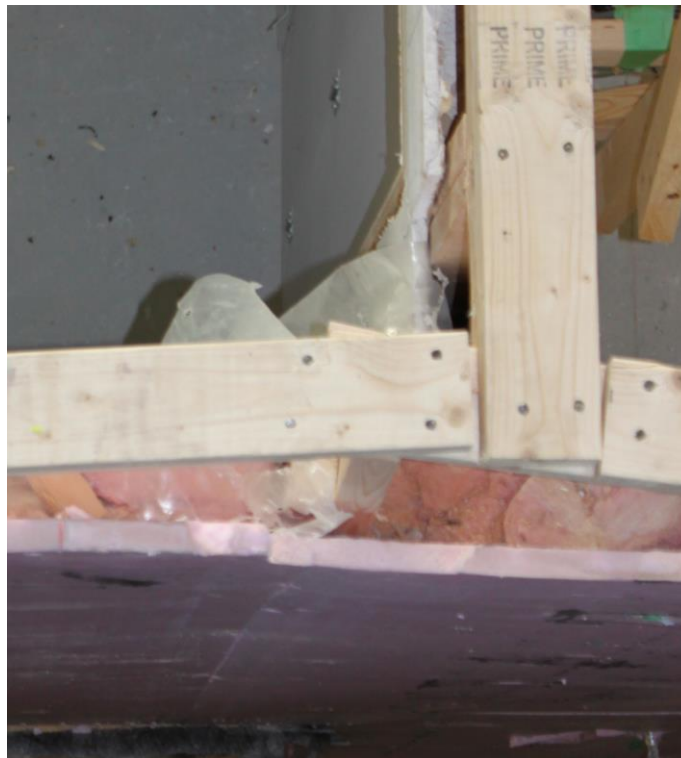
Figure 6.6 – Minimal top plate overlap located at D1.
