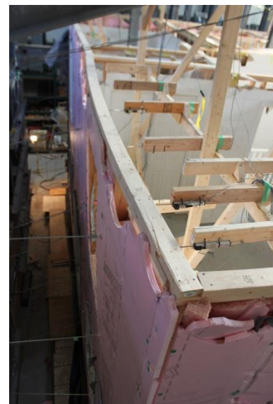
Figure K2 - North wall looking from the West during the test with no brick veneer
