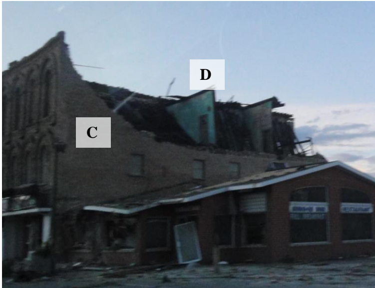
Figure 1.4 -A damaged structure in Goderich, Ontario. Picture courtesy of Sarah Stenabaugh
