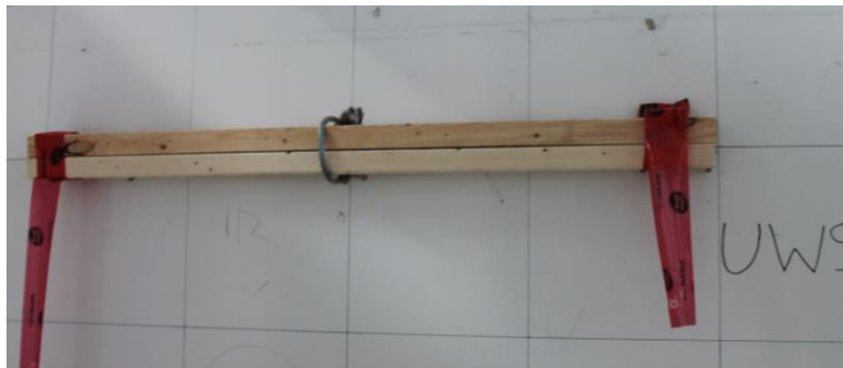
Figure 3.7 - A wood spreader beam installed at B10, on the second floor, set up to apply negative pressure (outwards loading).
