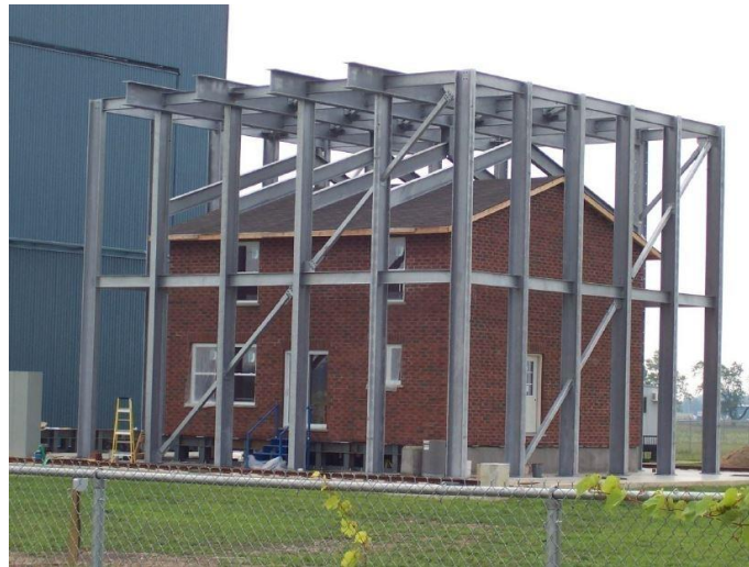
Figure 3.1 - The 3LP test house with the gable roof still in place viewed from the North West looking towards the South East. With reference to Figure 3.2, the main wall with windows which can be seen is wall A1-J1.
