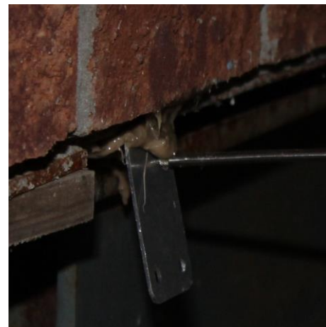
Figure A14- Close up of the DT connection to the metal plate at the base of the house
