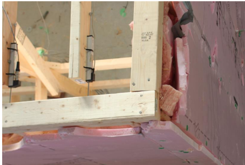
Figure 7.1a - The corner located at A1 with no brick before loading.
