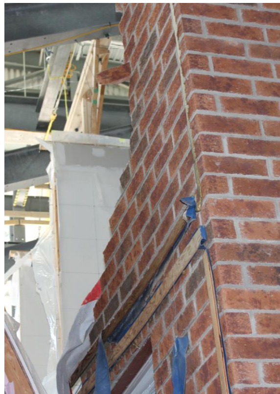
Figure 4.3 - Damage to the house similar to what was observed in Barrie and Goderich.
