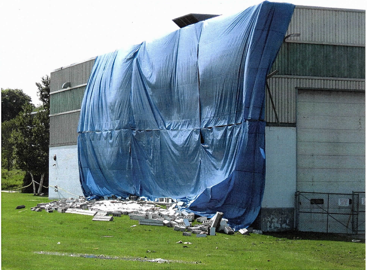
Figure 9: Baytech Plastics located on Hwy 12 east of Midland. Picture taken in a NW direction showing the outer cinder block wall that had sustained severe damage and partial collapse. The upper portions of the warehouse had evidence of siding removal
