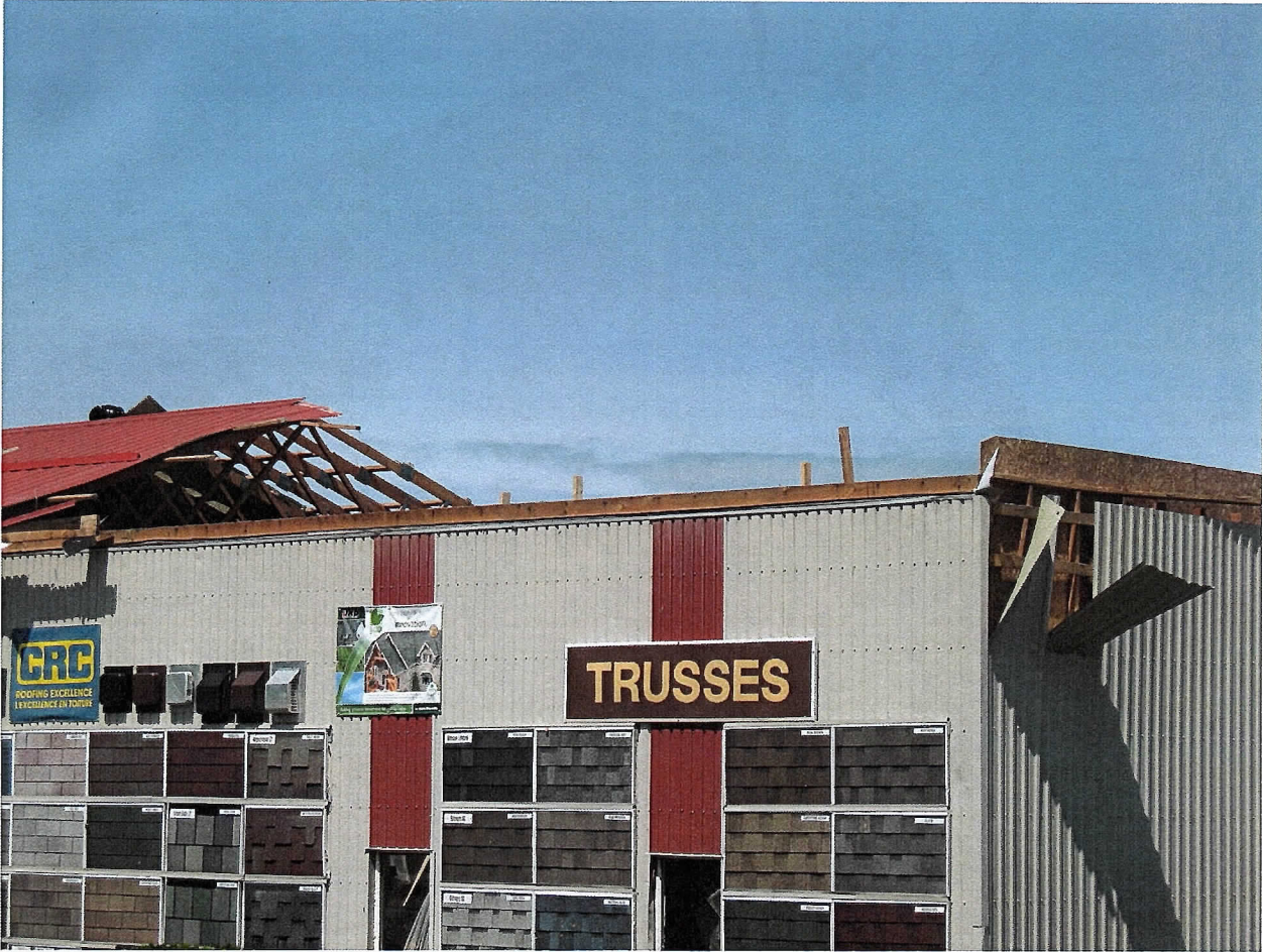
Figure 10: Sargeant Fuels industrial compound. Picture taken towards the northeast showing the removal of roof frame structure and metal plating.
