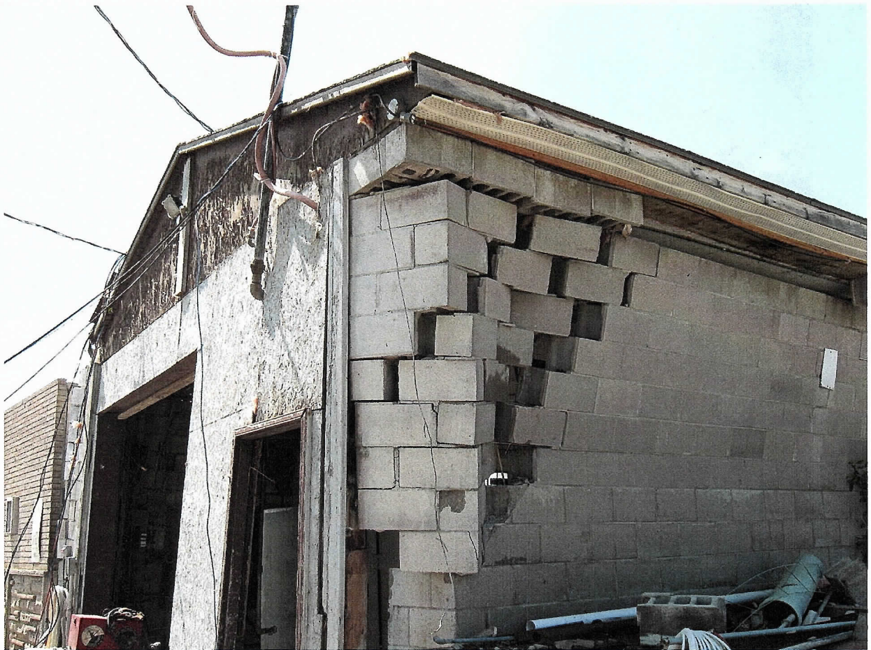
Figure 11: Southern building of the Sargeant Fuel industrial compound found on Hwy 93. Picture looking northward showing the dislodged roof from the cinder block masonry walls. Notice that some of the cinder blocks maintained contact with the roof while
