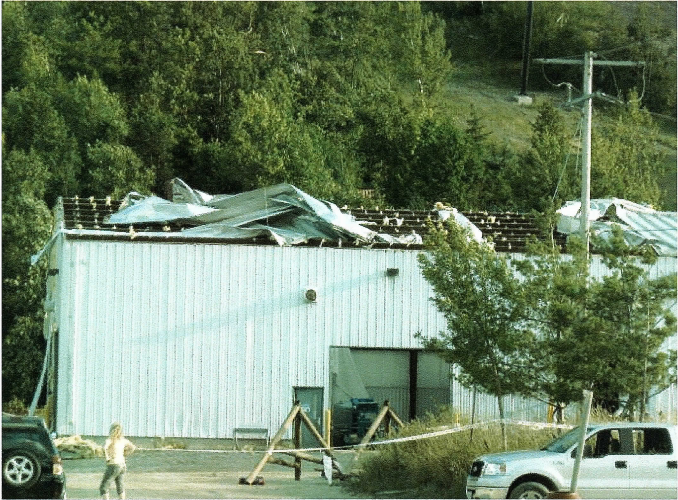
Georgian Peaks Ski Resort - Damage to storage building - looking south
