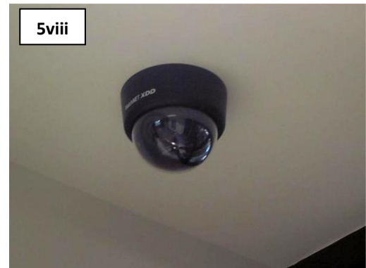
Security camera at the Cornish Library. (Photo by author.)
