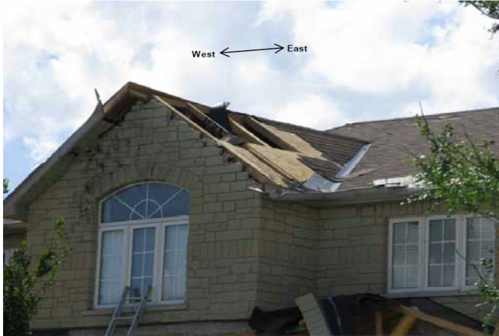
Figure 1.3 Shingle, sheathing and flushing loss on the upper roof (August 20, 2009; Vaughan, Ontario; photo courtesy of G.A. Kopp).
