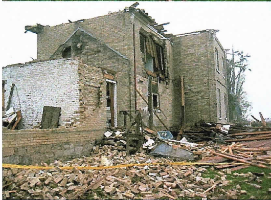
Looking W at the rear of the house where a portion of the 2nd floor triple bricked wall has been destroyed. The back of the house which was completely destroyed was old single brick. Large tree also uprooted.
