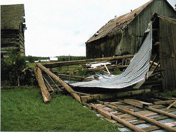
Figure 7: machine building completely flattened near waypoint 009 on figure 3.
