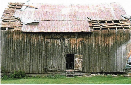
Figure 6: damage to barn roof near waypoint 009 on figure 3.
