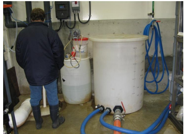
Reactor Trains A, C Exit Connections at the Flow Rate Measuring Tank.
