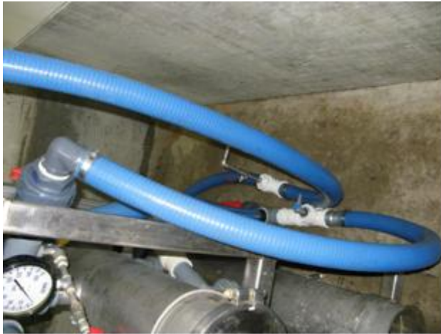
Reactor Trains A, C Exits.
