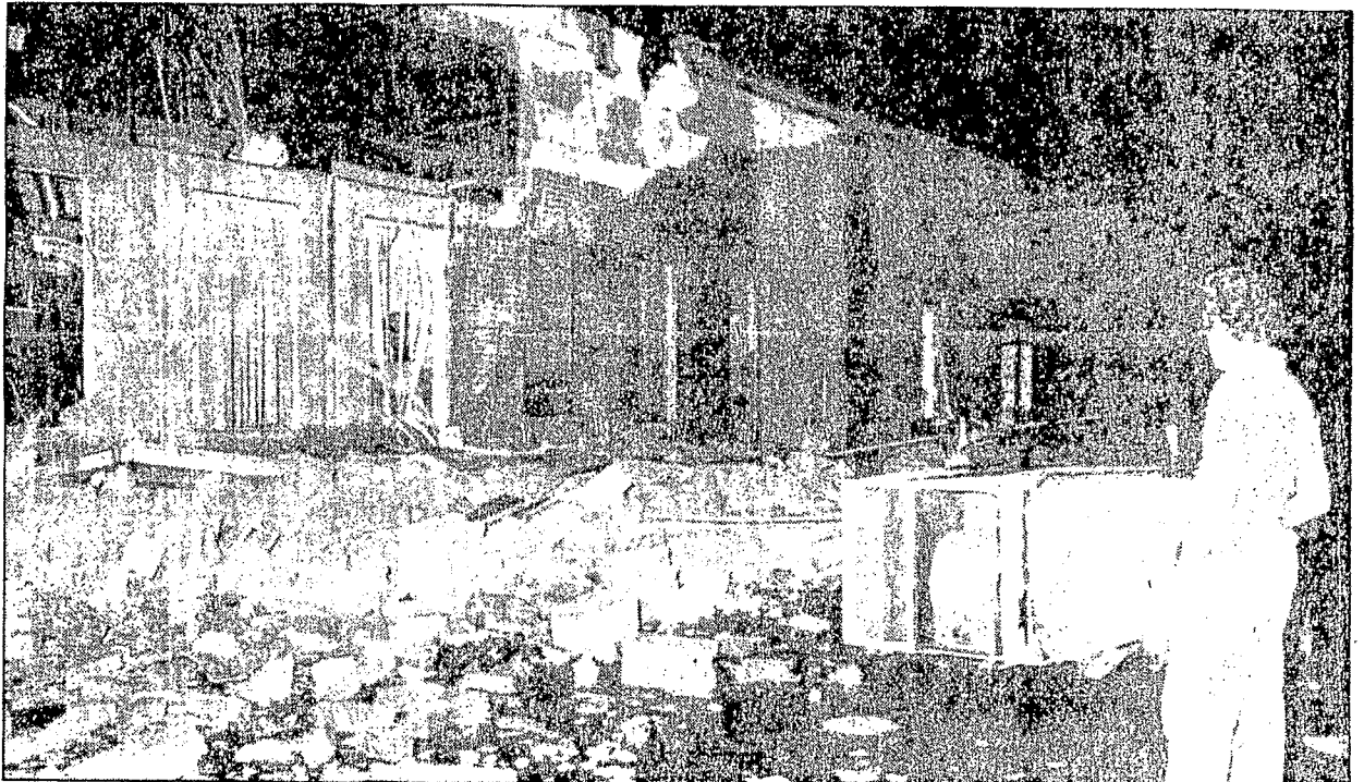
Business hit: Allen Snow, an employee at the Bedford Bedding and Upholstery Ltd. plant, surveys the damage at the Weston Rd. factory hit by last night's high winds, which destroyed part of the building, ripped the roof off
