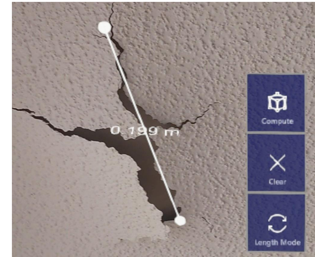
Figure 6: Length measurement of a crack using HL2
