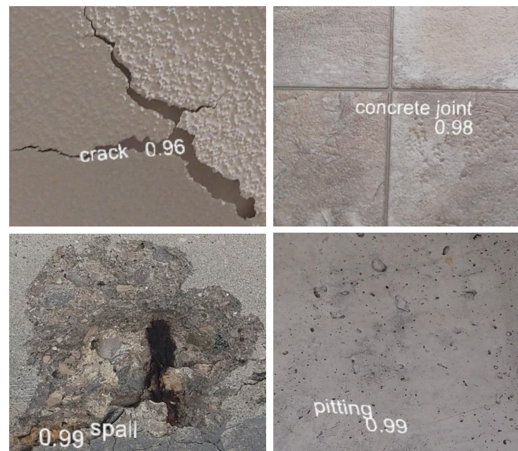
Figure 5: Classification result of four classes (crack, concrete joint, spall, and pitting) using HL2
