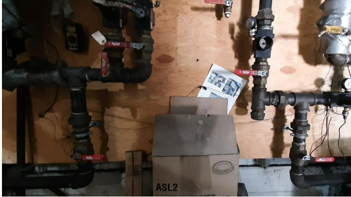
Figure 23 - The bottom left red handle is to be opened and closed for gas entry into the vessel.
