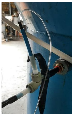
Figure 21 - T-tube connection with pressure transducer hoses passing through it to reach the backflushing system and the atmosphere. Since this assembly was constructed with materials on hand, possible alternatives can be used to simulate the same process.
