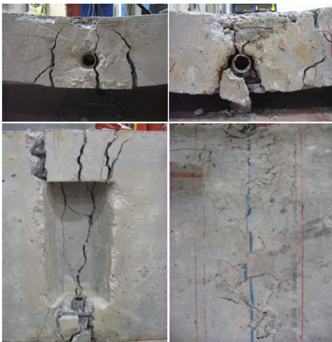
Figure B-6 Failure profile (the uncoated segment, Test 2)
