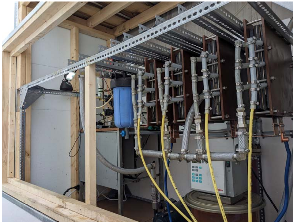
Figure D Pilot scale BioGenerator fuel cell bank (exterior).
