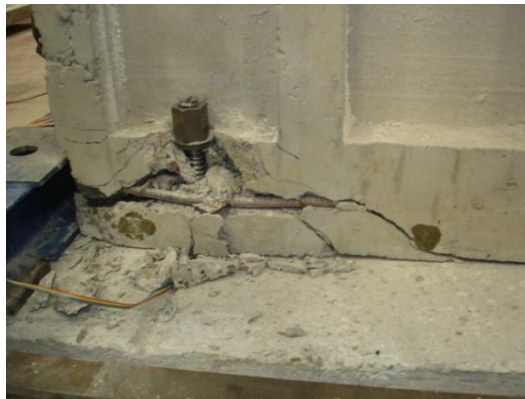
Figure 2.16: Extensive damage in the concrete surrounding the tension anchor (post-peak)
