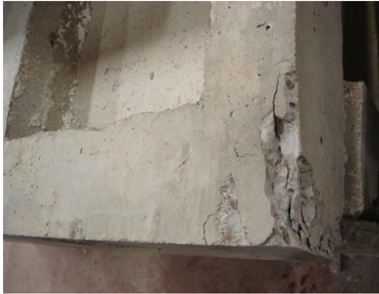
Figure 2.28: Cracking and spalling of concrete at the compression toe
