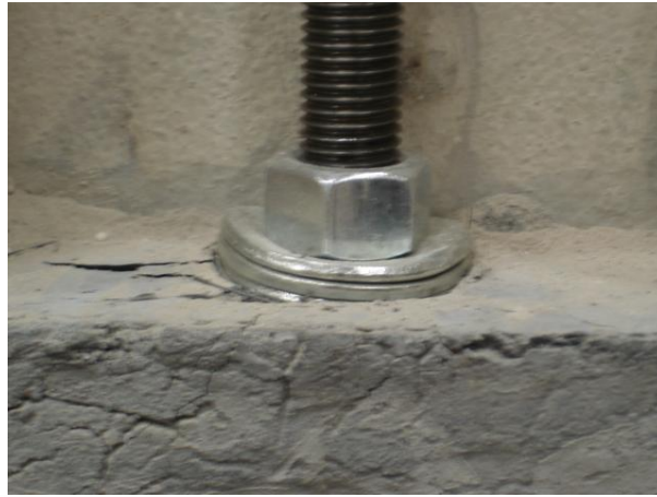
Figure 2.40: Cracks in the anchor block area
