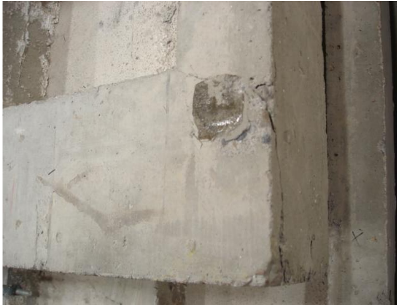
Figure 2.33: Cracking and spalling of concrete at the compression toe (Test 3)
