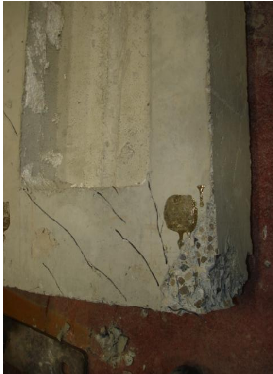
Figure 2.41: Concrete compression failure
