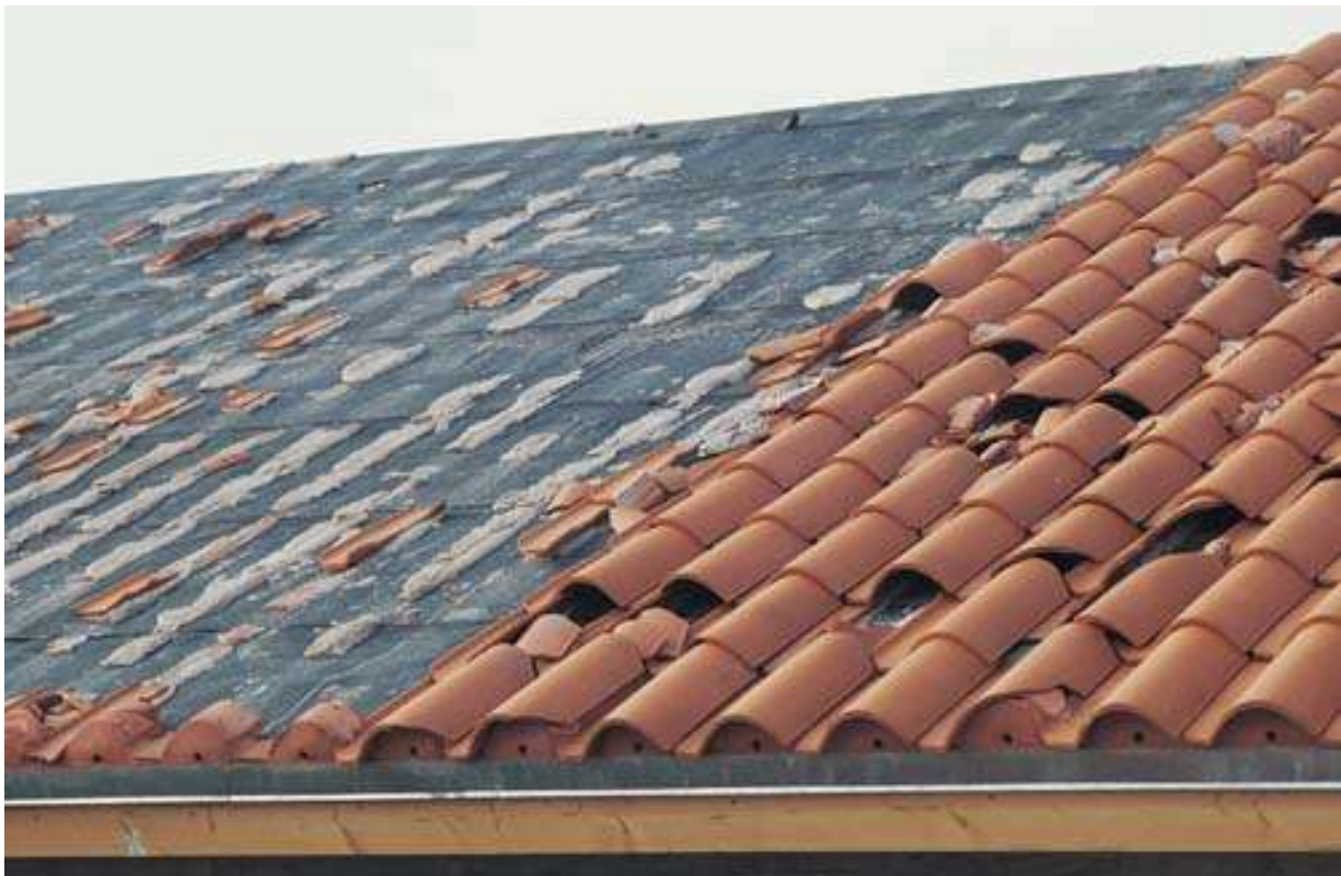
Figure 6 - After Hurricane Andrew 1992. These clay tiles were mortar-set. Three failure modes are illustrated: Separation of the mortar from the cap sheet, separation of the tile from the mortar and debris impact damage (photo courtesy of TLSmith Consulting Inc.).
