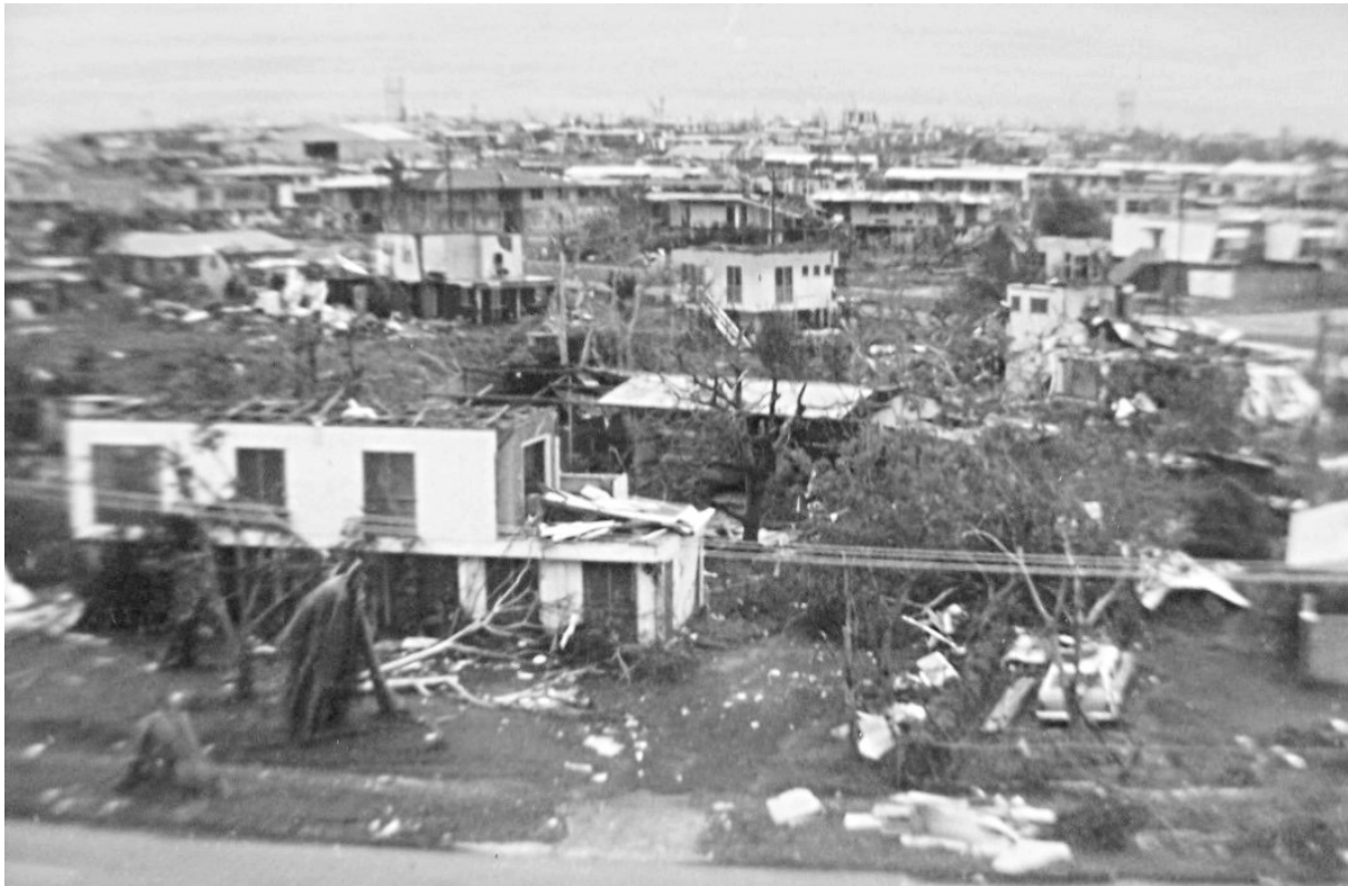
Figure 5 - Damaged houses after the passage of Cyclone Tracy on Christmas day 1974 in Darwin, Australia (Wikimedia Commons).
