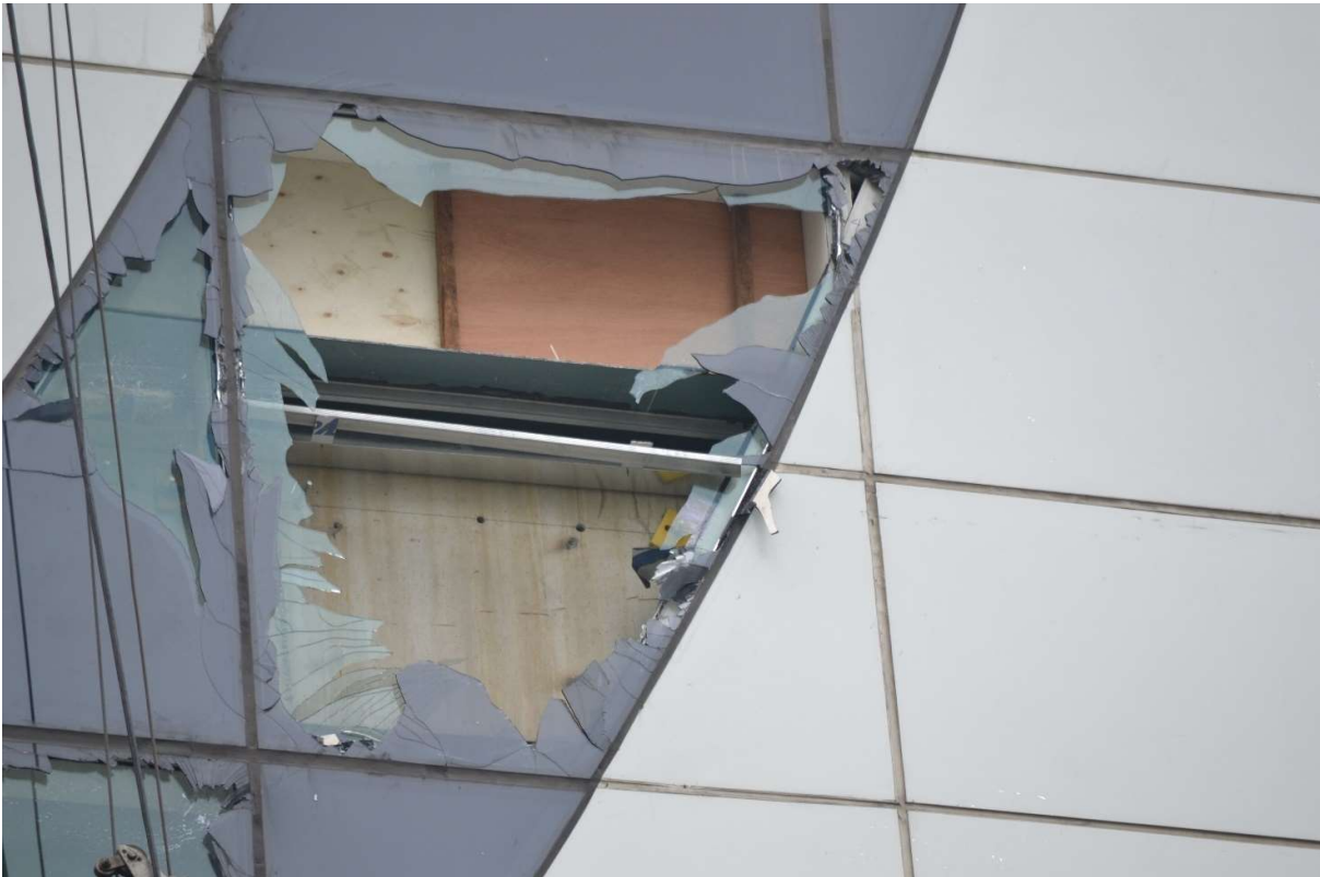
Figure 8 - Manila, 2016. When Typhoon Glenda hit the Philippines capital in 2016, building envelopes have been heavily damaged, especially the glazed panels, due to wind-borne debris impact (photo courtesy of Joe Khoury).
