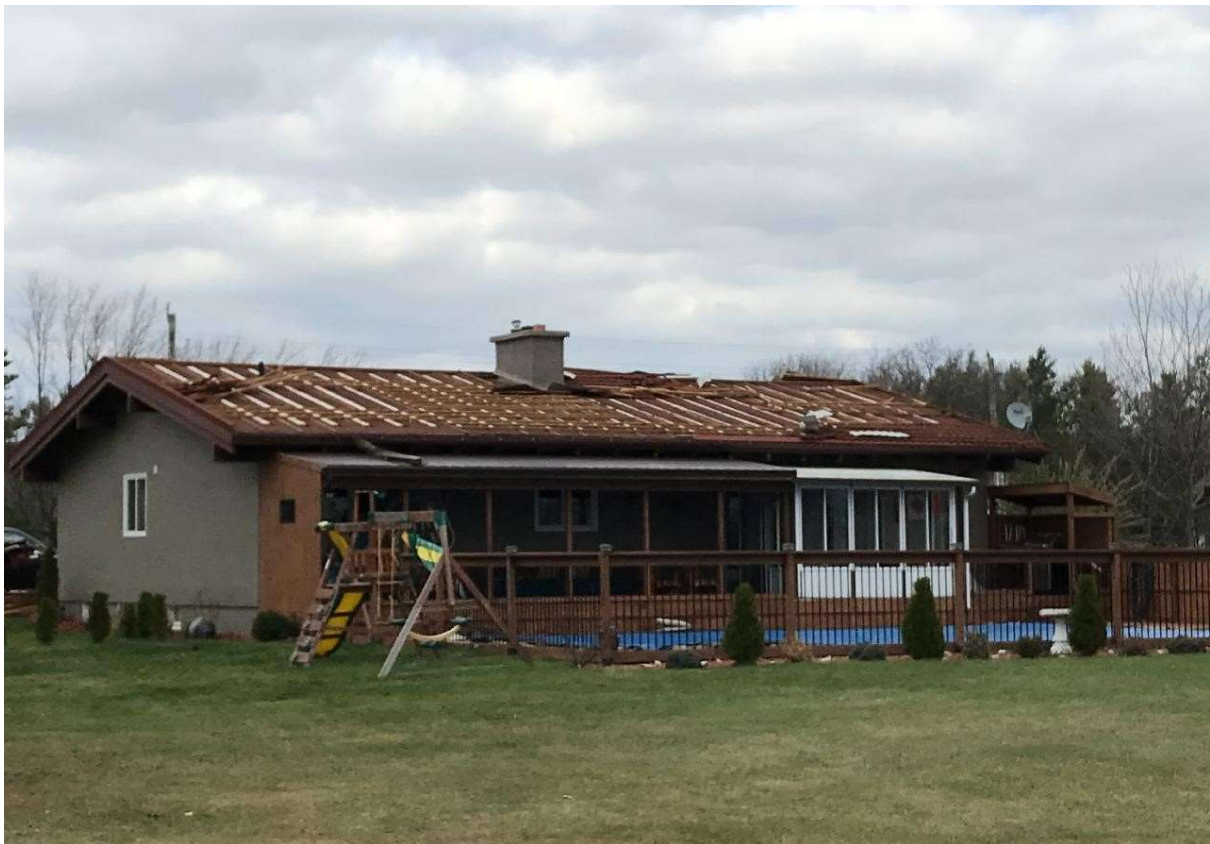
Figure 3 - Downburst winds in Dunnville, Ontario, Canada. November 11 th , 2020. Roof tile failure was recorded (Northern Tornadoes Project 2022).
