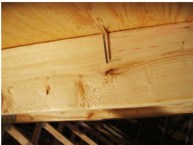
b) The typical improperly installed nail
