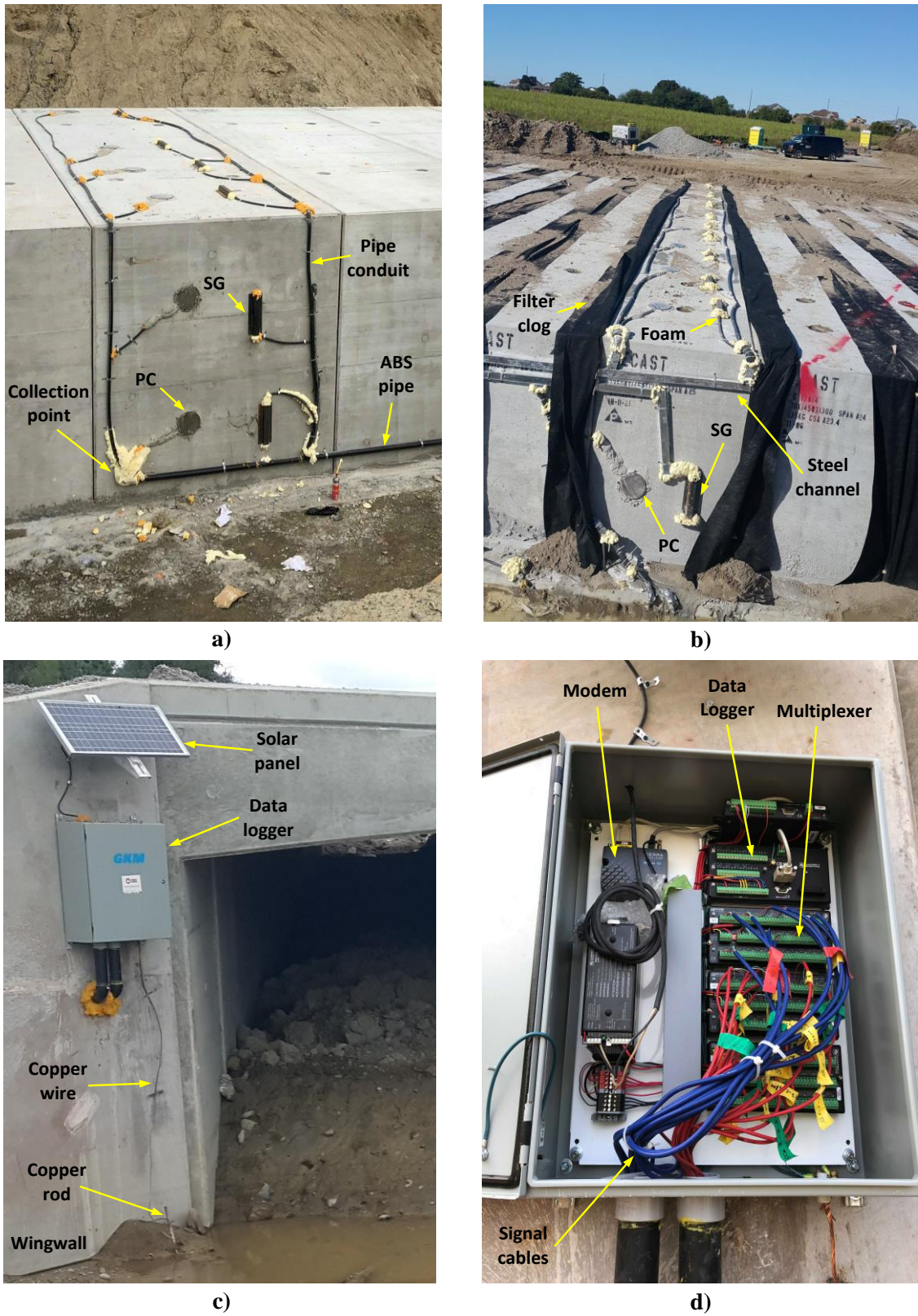
Figure 3-10. Overview of the final instrumentation: a) Remembrance culvert; Oshawa culvert; c) data logger and grounding system; and d) data logger components.
