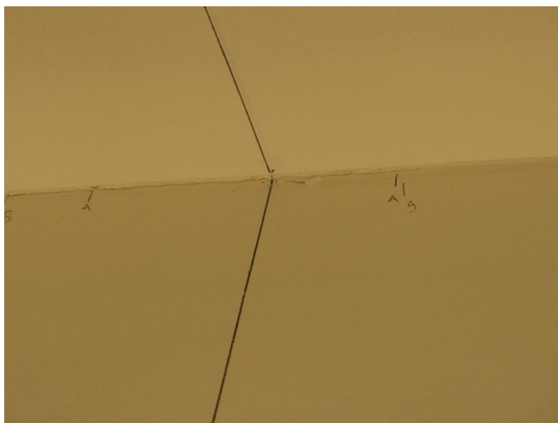
Figure 6.23 Cracks in the drywall below RTWC “S3”. Only minor hairline cracks are observed despite the damage that has occurred to the toe-nail connection directly above it.
