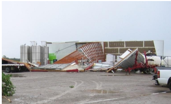
Figure 8.1 Picture of the Building facing South just after failure
