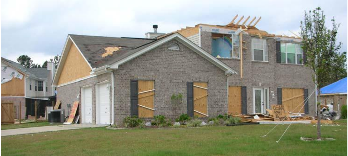
Figure 1.2 Failure of windward windows, shingles and roof trusses during Hurricane Katrina in August, 2005.
