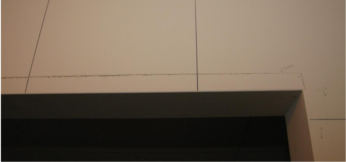
Figure 6.24 Largest crack documented in the test house, which was not the result of structural testing. Distance between vertical black lines is 0.3 m.
