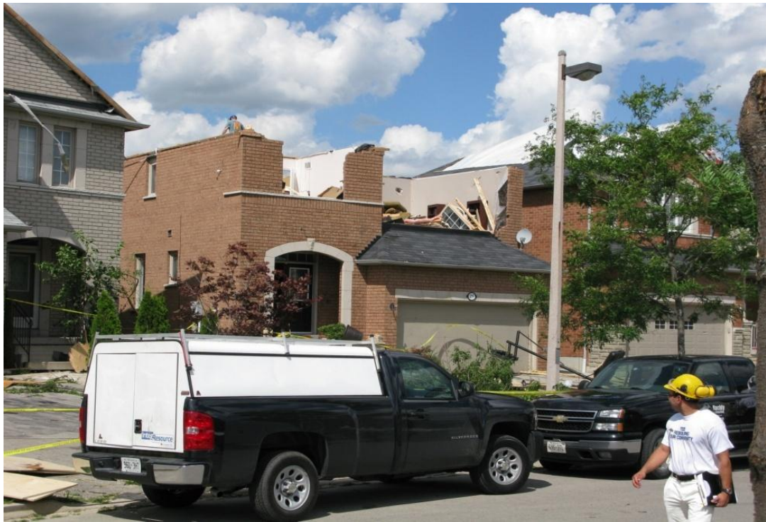
Figure 1.1 Global roof failure of a house due to a tornado that struck Vaughan, Ontario on August 20, 2009.
