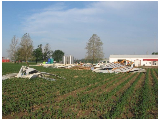
Figure 8.2 Picture of the debris field looking west towards the building
