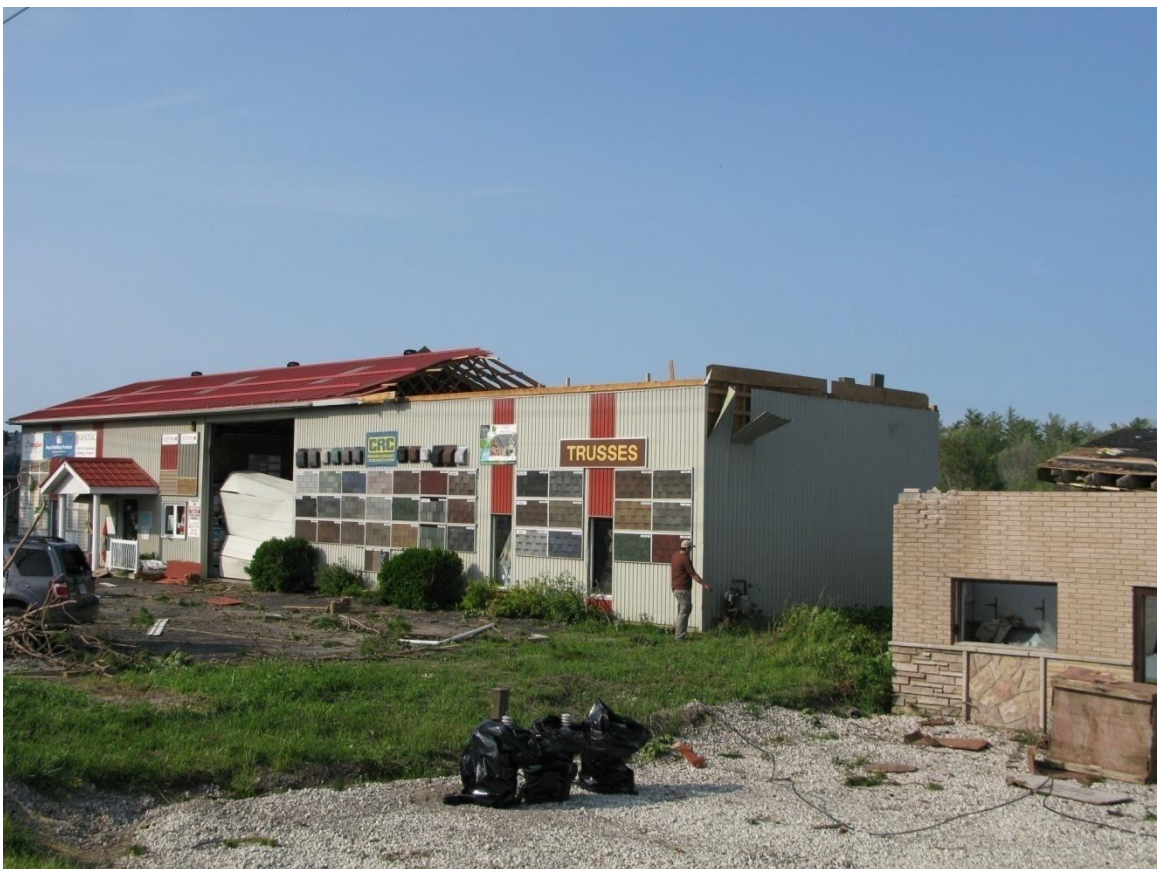
Figure 1.3 Failure of a group of trusses during a tornado in Midland Ontario, June, 2010.
