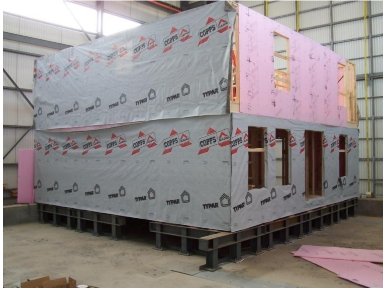
Figure 2.3 Photograph of the test house under construction. Photograph shows the house prior to the installation of the brick veneer and roof trusses.
