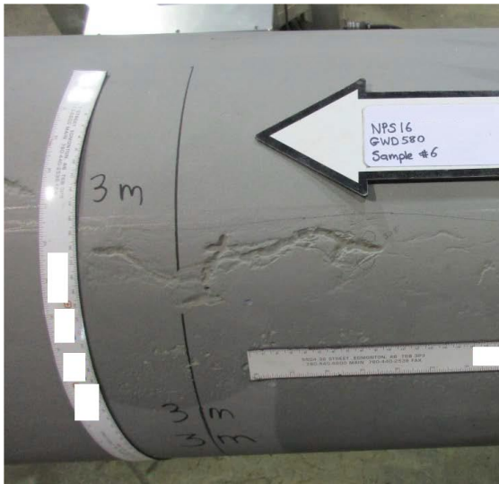
(a) Naturally-occurring corrosion defect on pipe specimen 16-6
