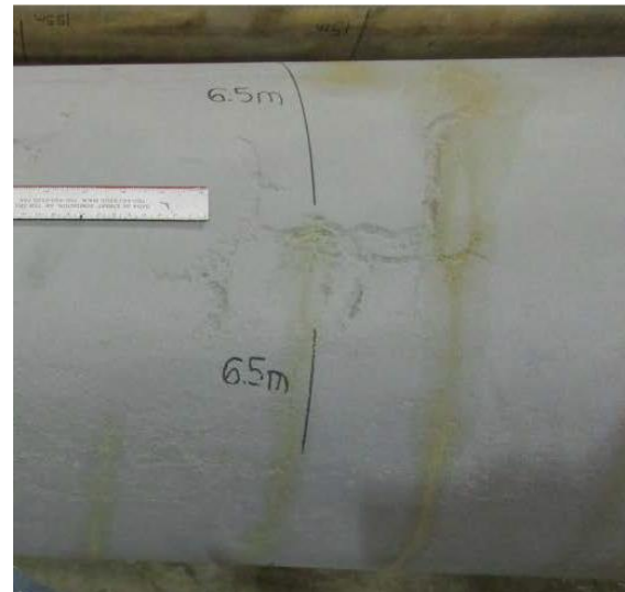
(b) Naturally-occurring corrosion defect on pipe specimen 16-7
