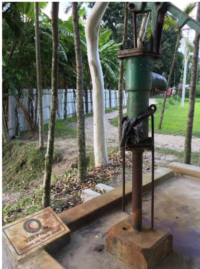
Figure 12: Tube-well provided by the Red Crescent
