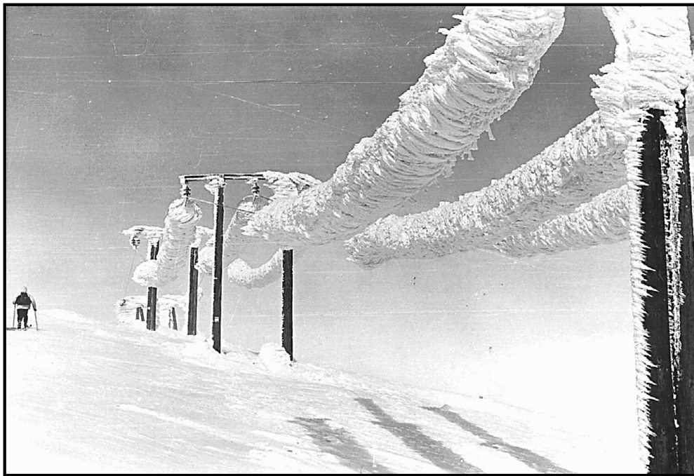
Figure 1.1. 305 (kg/m) of rime ice accumulated on an overhead line in Norway the 18 th of April of 1961 (Makkonen, 2000).
