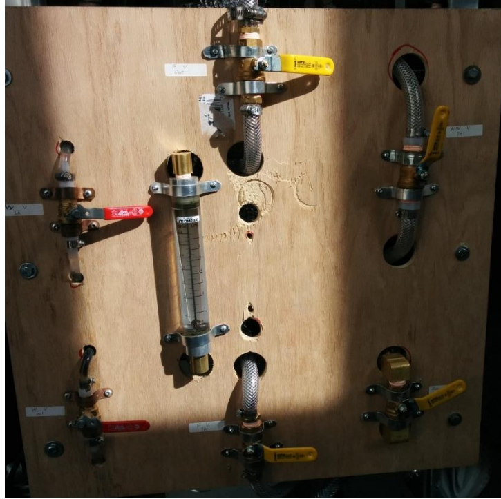
Figure 3.4 Hydraulic control valve
