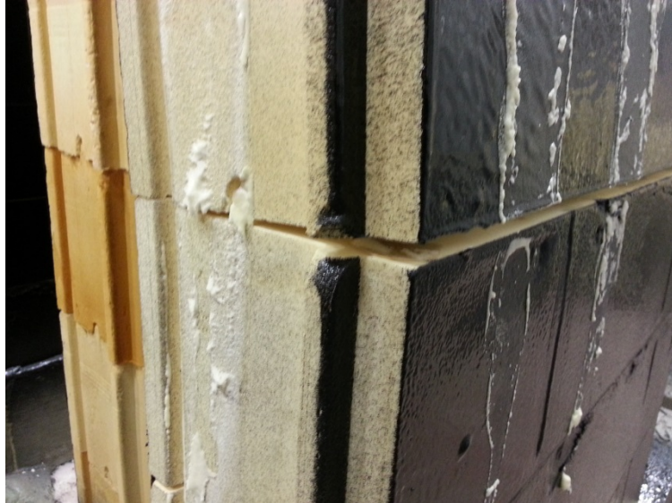
Figure 5.11: Block separation due to expansion of the FPF
