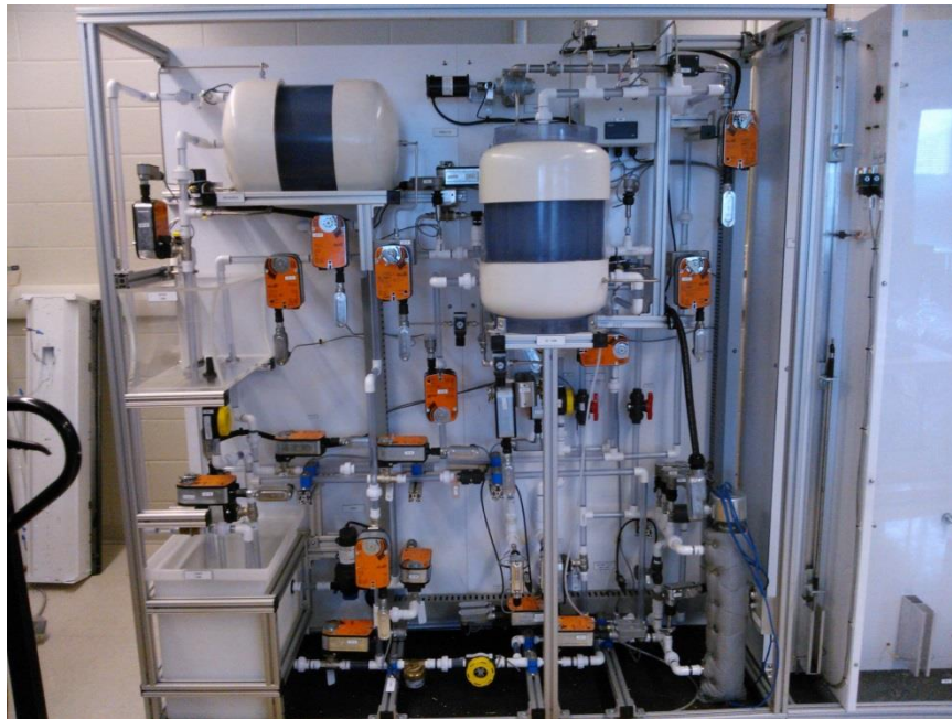
Figure 3.12 Field devices of NPCTF
