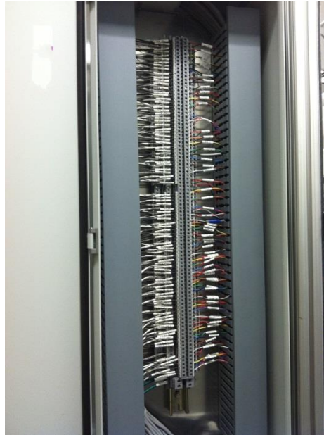
Figure 3.11 Wiring of DCS cabinet
