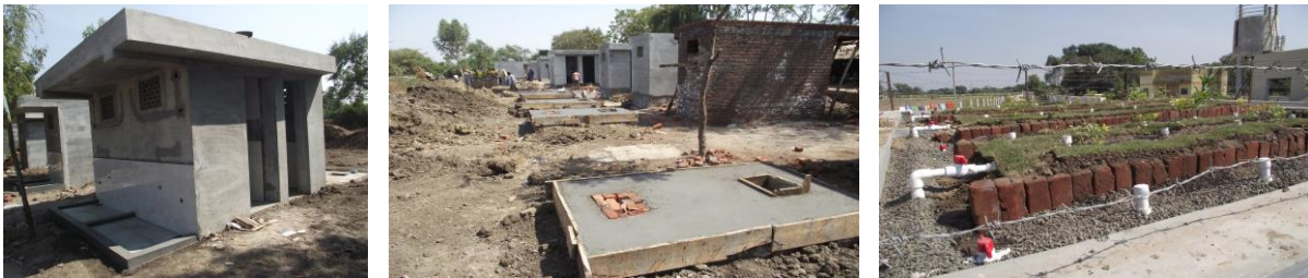
Figures 4, 5 & 6: Construction of toilet and bathing facilities, interceptor tanks and constructed wetland in India
