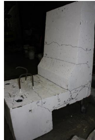
b) Crack pattern at the right side of the specimen
